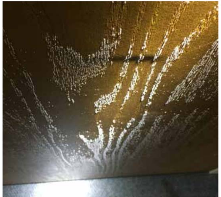
Mold on a wooden door. Tim Popp said if you are looking for mold, start looking at things that are at a four-foot level and below.
