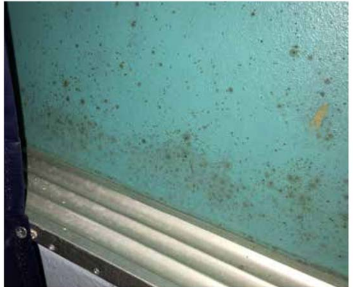
Bulletin boards are not exempt from mold.
